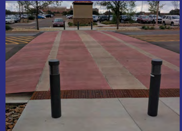
A "tabletop" pedestrian crossing which maintains the pedestrian walking surface and bollards used to separate vehicles from pedestrians.
